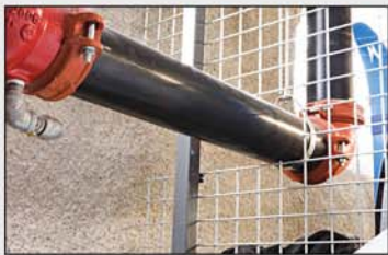
cut-outs around pipes
