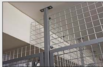
cut-outs around vents
